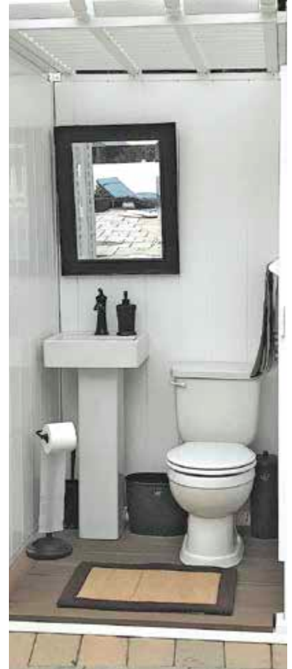
Outdoor shower stall and bathroom in a typical installation.
