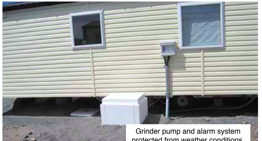
Drainpipe from trailer leading into a Sanicubic 1 grinding system
