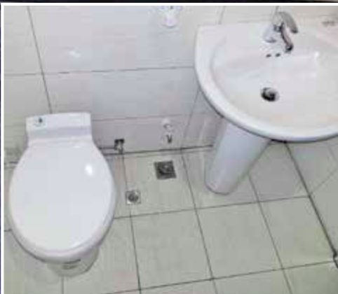
Sink connected to Sanicompact macerating toilet and pump system.
