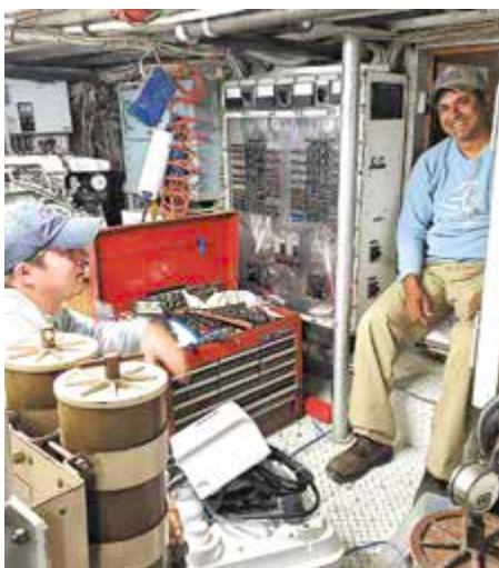
Dr. Rusty Day (left) and installer Ronald Rampersad (right) in the RV MANTA's mechanical room. The Sanicubic being installed is in the foreground, center.
