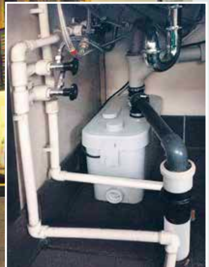
Sanivite installed underneath the counter sink
